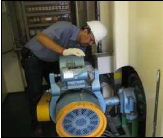
ELEVATOR VISUAL & FUNCTIONAL TESTING INSIDE THE MACHINE ROOM
